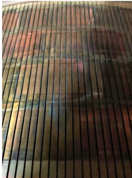
Figure 2: Excessive heavy loads, high current at low RPM for long periods of time
