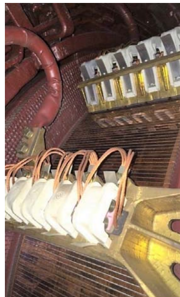
Figure 11: Acceptable condition, medium film
